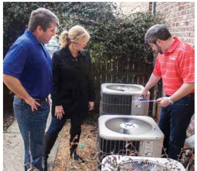
GreyStone members Scott and Kathy Patman learn how to reduce electricity costs by caring for their HVAC units.
